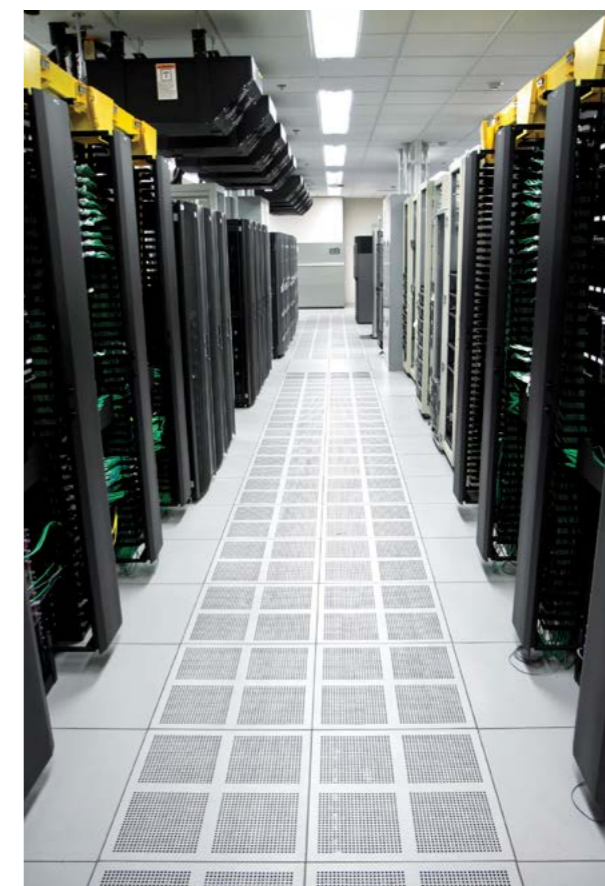
Datacenter • Bron: DDA-interxion
